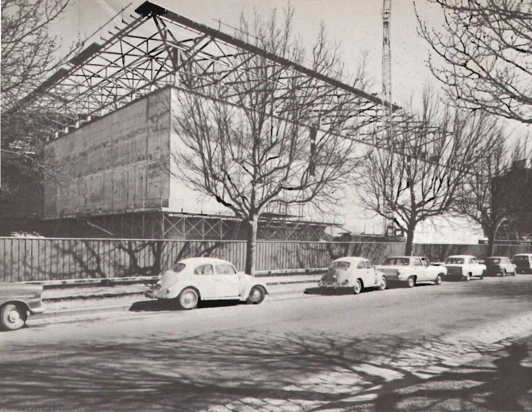
South-east corner of the Gallery illustrating extent of elevation and steel structure of eaves. [National Gallery of Victoria]
