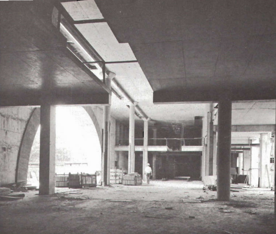
A view of the progress of the main archway and entrance hall. [National Gallery of Victoria
